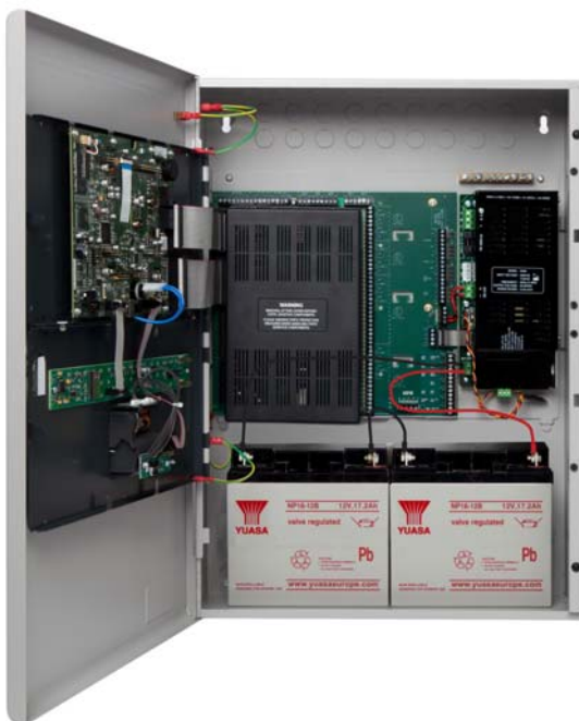
Figure 2-11 Connecting Standby-Batteries of the 5.25 Amp Power Supply
